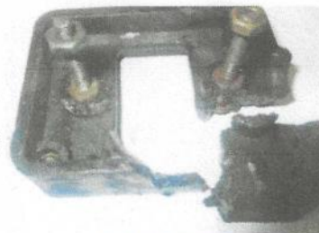
A truly terminal terminal-box
